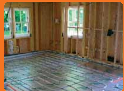
Typical UFH installation
